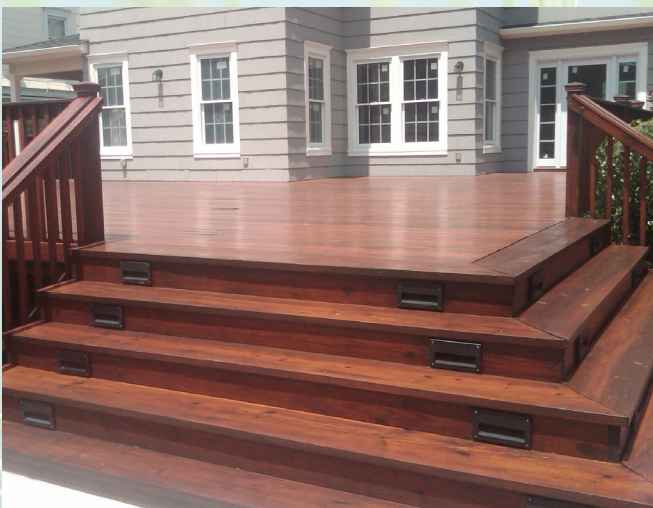
Power wash winter leftover debris on your deck or patio to make your outdoor living room sparkle.
